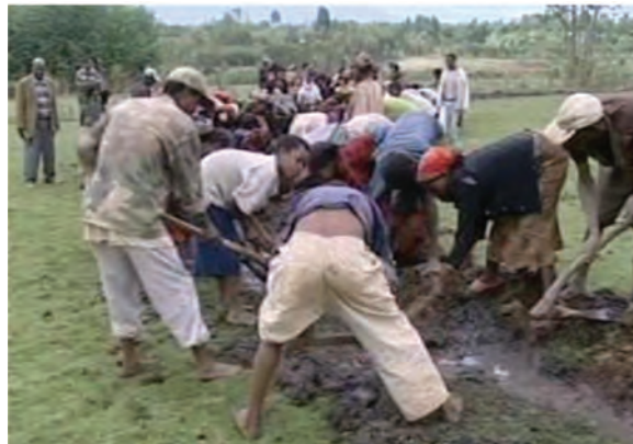
Figure 9.1 Community members digging a ditch to drain mosquito breeding pools. (Photo: Dr Daddi Jima)
